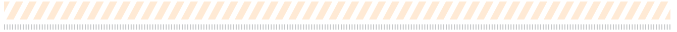
TRULINE® wall system being installed to help control erosion and save homes on the beach in Northeast Florida. Photo credit: TRULINE.
